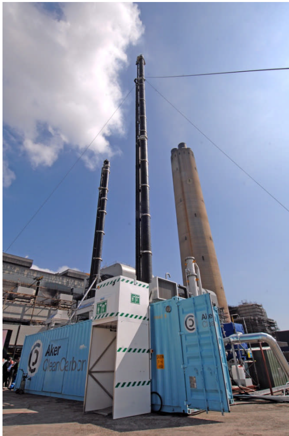
Mobile Test Unit, Longannet Power Station
